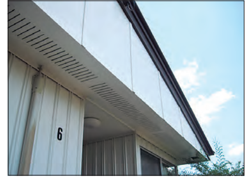
Asbestos cement sheet to a Gable wall
