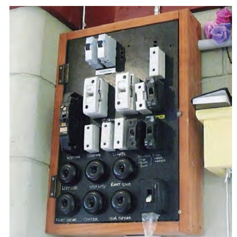
Asbestos based resin Electrical fuse board
