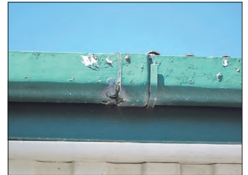
Deteriorated Asbestos Cement gutter
