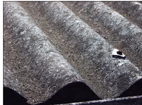
Close up of poor condition corrugated asbestos
