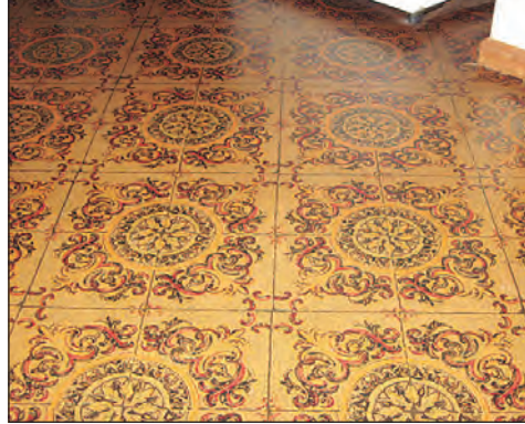
Asbestos backed vinyl
