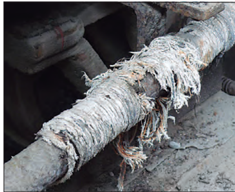
Asbestos rope in poor condition
