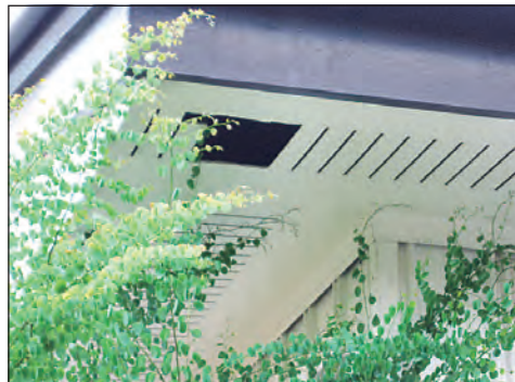
Damaged A/C sheet slotted eaves
