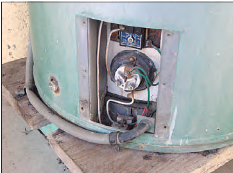
Asbestos Millboard inside Hot Water Service
