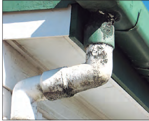
A/C gutting & down pipe
