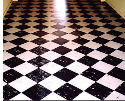
Asbestos containing vinyl tiles
