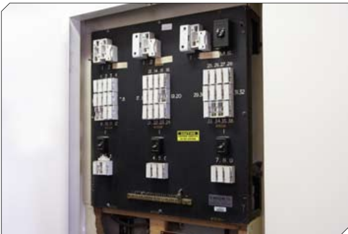
Figure 16: Asbestos-containing zelemite electrical switchboard panel.
