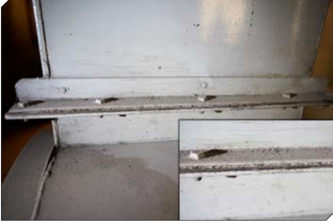
Figure 14: Asbestos rope seal in duct joint with close-up inset.
