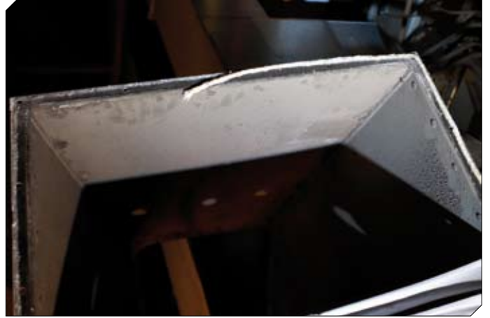
Figure 15: Detached asbestos rope seal and remnant debris on duct.
